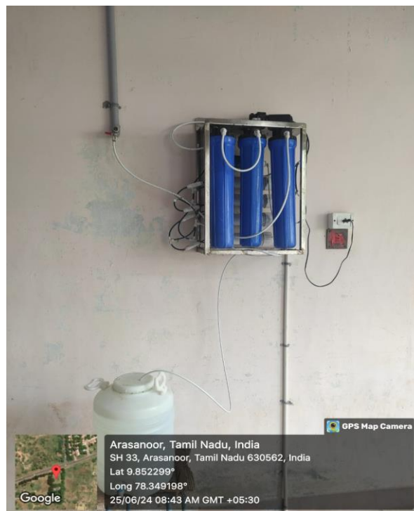
WATER PURIFIER IN HOSTEL
