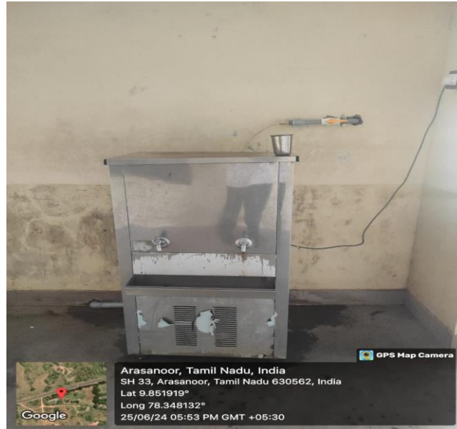
WATER PURIFIER AND DISPENSERS
