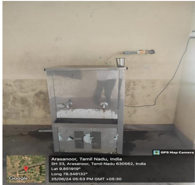
WATER PURIFIER AND DISPENSERS
