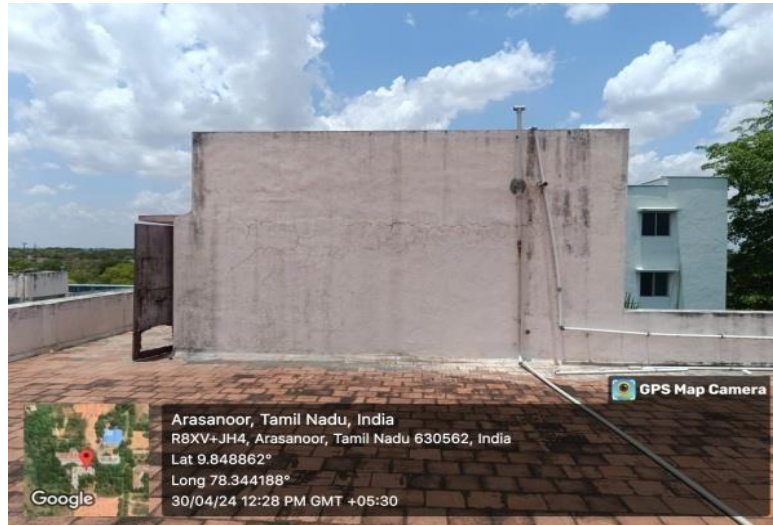
WATER STORAGE TANKS
