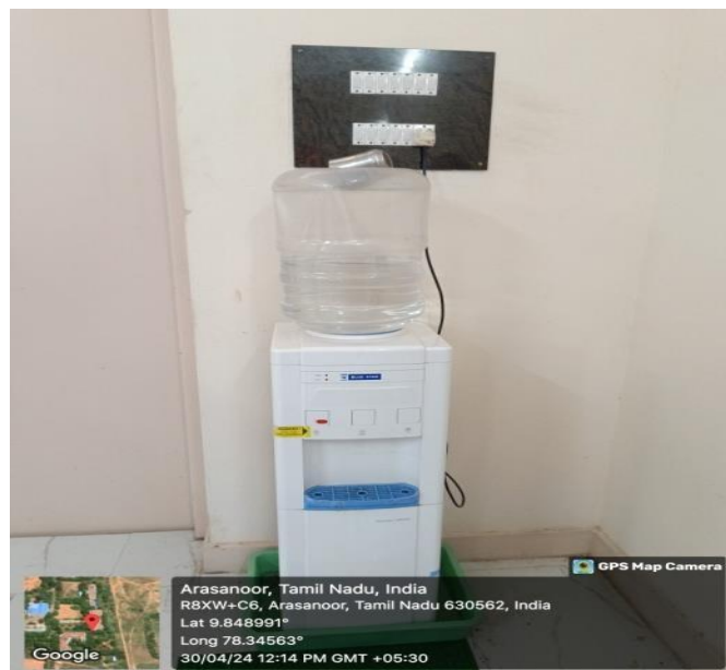
WATER PURIFIER AND DISPENSERS
