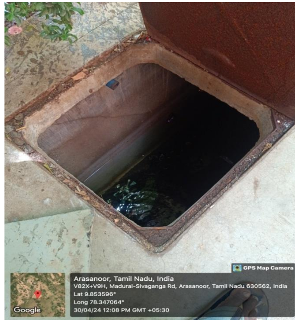
BORE WELL & SUMP
