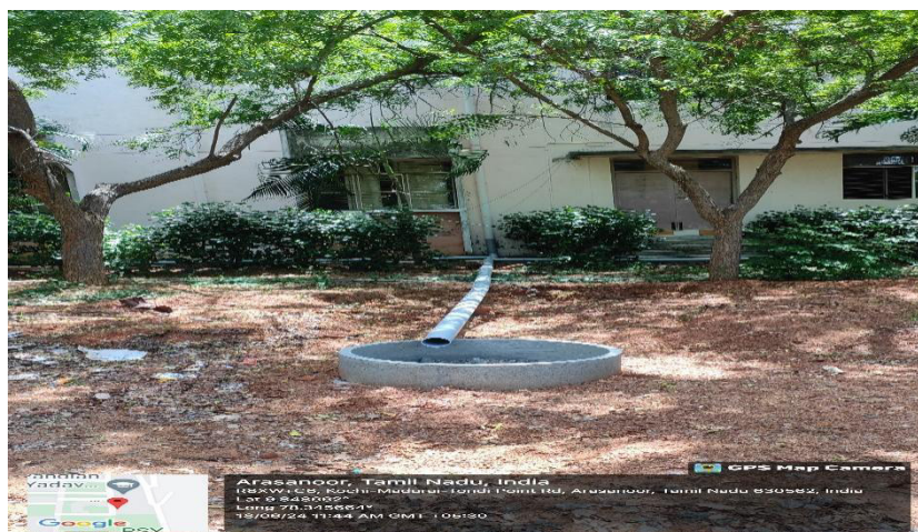
Figure 3: Rain Water Harvesting System
