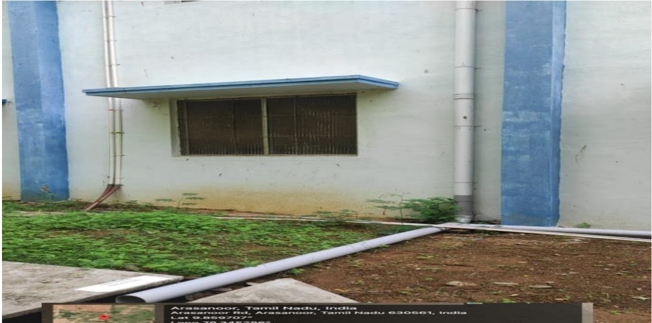
RAIN WATER HARVESTING
