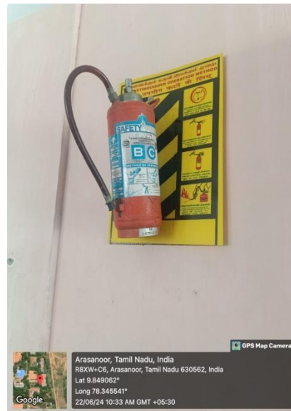
Fire Extinguisher at Admin block
